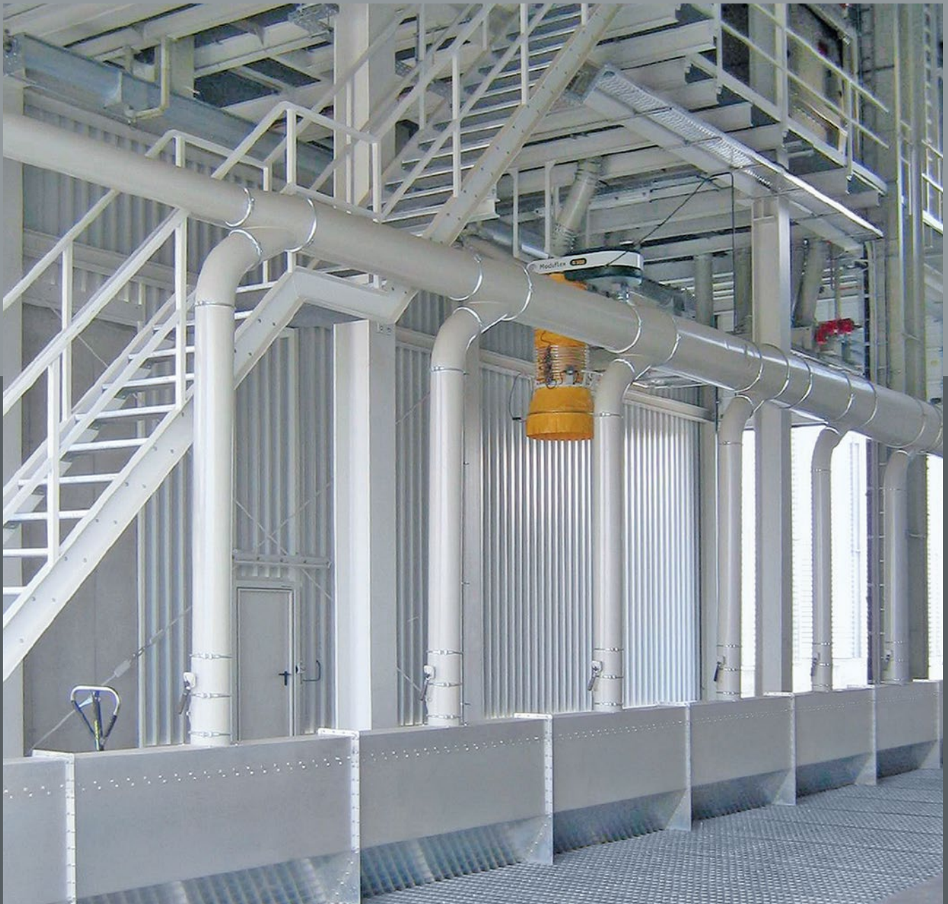
Grain input gutter 2.5 x 16 meters, with suction cascade and connecting pipe to a decentralised RUBERG jet bag filter.
